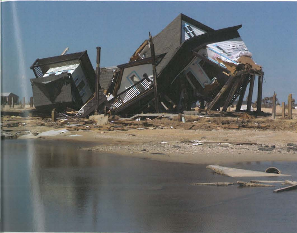
Flooding during Hurricane Ike in 2008 undermined tall posts supporting houses on the barrier island east of Galveston, Texas, toppling them into the surf.
